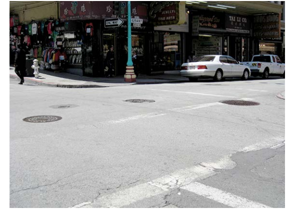
Faded Crosswalk markings
