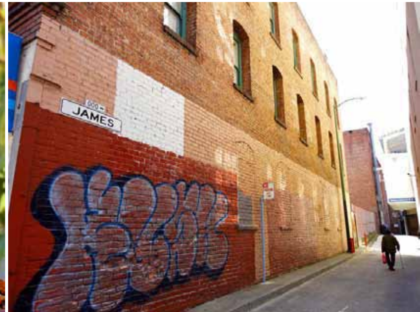
Figure 7.6. Current conditions of James Alleyway. This alleyway is both an entrance to a residential unit behind Chinese Hospital and to the hospital's parking structure on the right.
