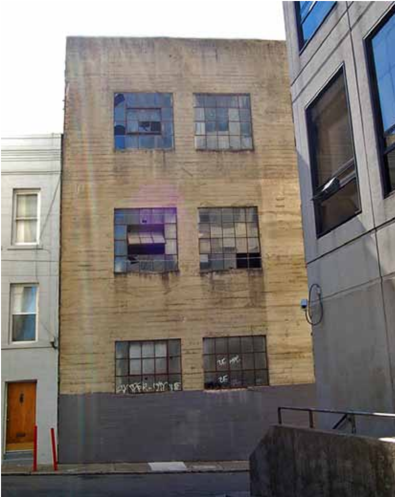
Figure 7.2. Broken windows and graffiti on a building in the middle of the alleyway
